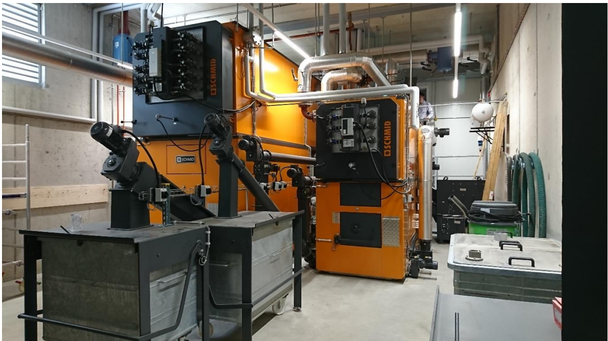
Figure 13: Example image of a 1.5MW and a 500kW biomass boilers
